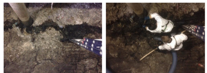
Fig. A2. Cleaning of the FOG layer at the Hoekersingel WWPS (source: municipality of Rotterdam).
